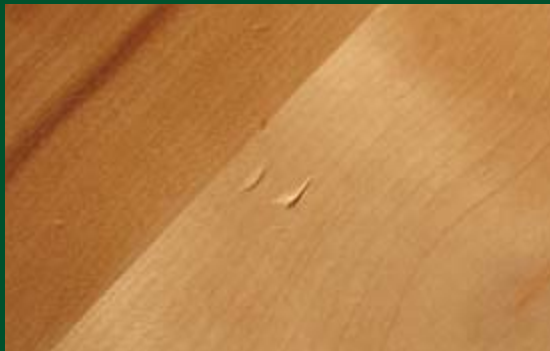
Dents (these usually require board replacement).
