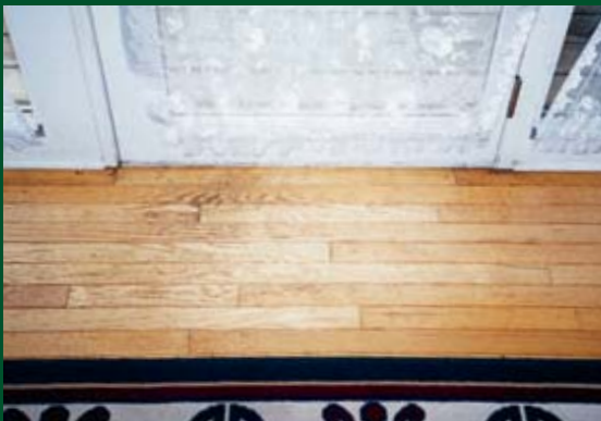
Dirty floors with finish totally worn off.
